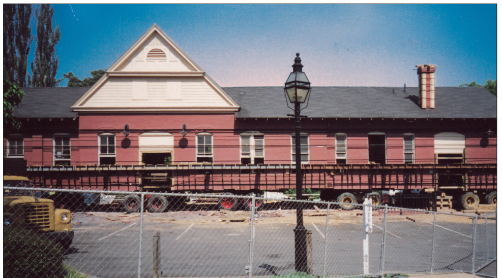
The simplest technology — wheel and board — moved the old train station to a new site.
